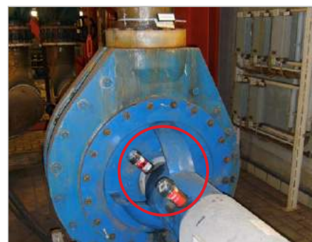
Lubrication of drive shaft on pump
