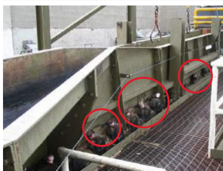
Bearing lubrication at the tree sorting system
