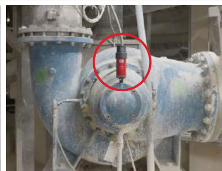
Pump bearing lubrication
