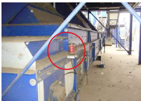
Lubrication of pillow block bearing on conveyor
